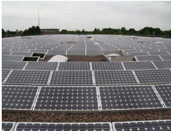
Bremerhaven Bus, Germany 738 kWp 4100 panels*180Wp
