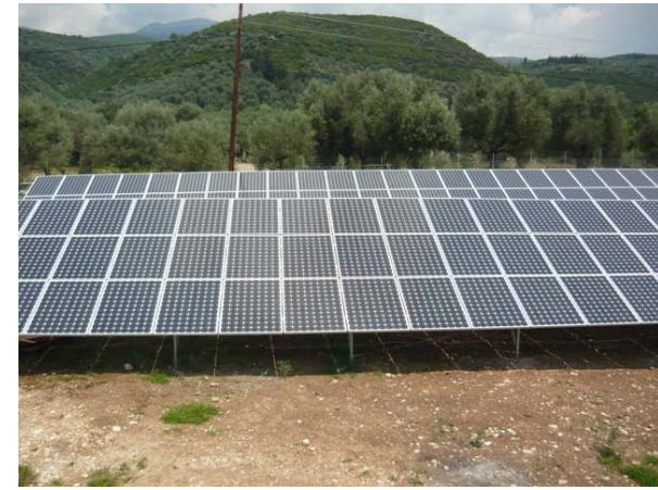
Agrinio, Greece 38.88kWp 155 panels*250Wp
